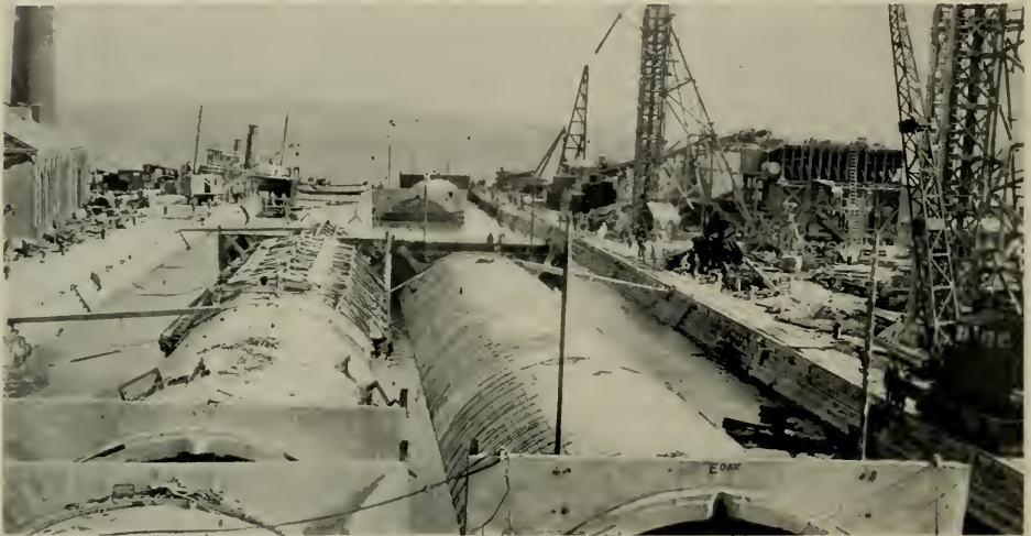
FOUR PRECAST SEGMENTS FOR GEO. A. POSEY TUBE Drydock Flooded for Removal of Completed Segment
