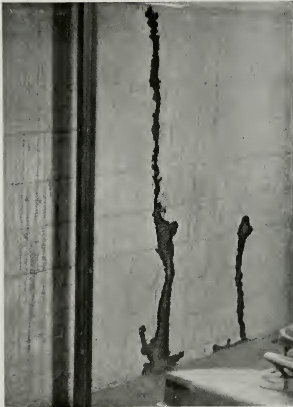
Fig. 22—Covered passageways composed of particles of earth and fragments of chewed wood, constructed by subterranean termites on vertical concrete walls for two stories in a heated warehouse in the San Francisco Bay region.
