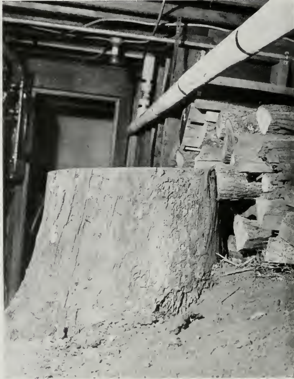
Fig. 21—Tree stump left under an apartment building. The stump is infested with subterranean termites. The firewood piled in contact with the ground and stump may also provide an avenue of attack.
