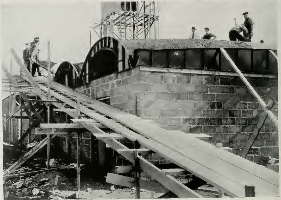
EXTERIOR VIEW OF REAR OR LAKE SIDE. NOTE STEEL GABLE FORMS. DOUBLE CURVE IS PLAINLY VISIBLE
