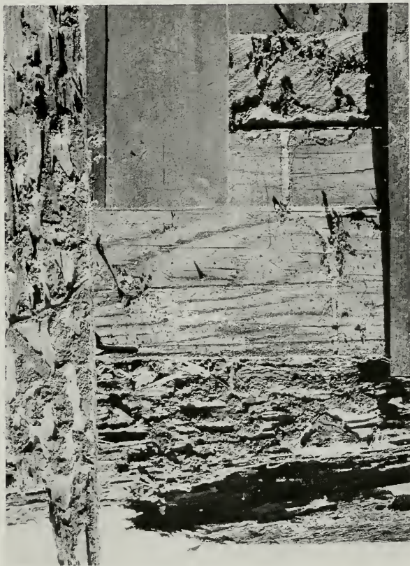
Fig. 24—Portion of the surface of a shingle-covered dwelling in Berkeley, California, after partial removal of shingles to show the surface attack on shingle-covered members and combined termite and fungus attack below. The shingles extended over the foundation to the ground.
