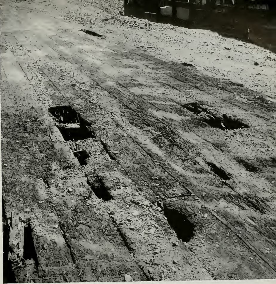
FIG. 2—VIEW SHOWING CONDITION OF REDWOOD COVER PLANKS, ISLAIS CREEK SEWER, AFTER FILL HAD BEEN REMOVED
