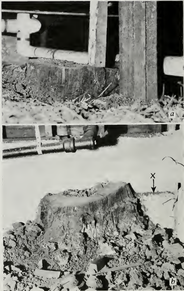
Fig. 25—Some causes of termite attack. a—Tree stump left under an apartment building. Examination revealed heavy infestation of stump by subterranean termites. A 4-inch by 4-inch post on the stump is a floor support. This provided the termites with a direct path to the joists. Intermediate post beside the stump rests on a concrete pier which has been covered with soil. Steam pipe helped to provide ideal conditions for infestation. b—Foundation wall built over tree stump. Part of stump also appears on outside of structure. Subterranean termites infested the stump. X indicates termite tubes from stump toward sill. As a means of getting rid of these infestations, holes should be bored in the stump and frequently filled with a preservative such as Reilly penetrating creosote until the stump is well saturated.
