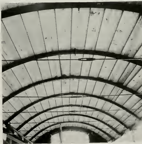
UNDERSIDE OF FORMS, SHOWING CURVED STEEL RIBS RESTING ON CURVED BEAMS—SHEATHING BOARDS—AND PLYWOOD SHEETS.
