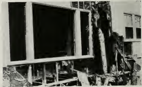
Fig. 4—The collapse of the wall and entrance of this home showed it to have been gutted by termites
