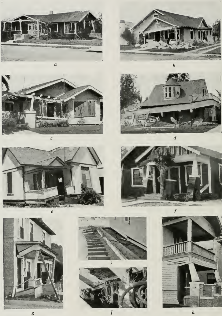
Fig. 1—(a-h) Typical examples of serious damage to frame houses at Long Beach and Compton, California, in the earthquake of March 10, 1933. Many of these failures were, in part, due to termite damage to under-pinning, as shown in details, i-j. The use of proper construction and wood, not attacked by termites, and fungi, would have prevented all but minor damage.
