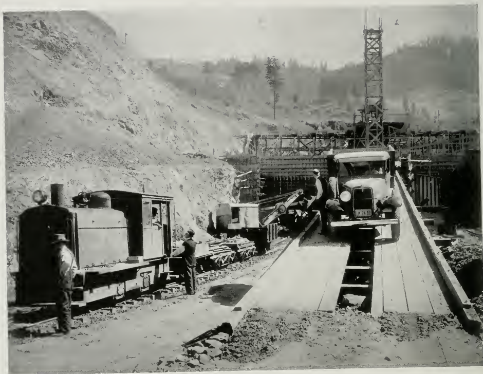
SPEED WORK ON HUGE CONTRA COSTA TUNNEL PROJECT Here is a section of the Broadway low-level tunnel project, near Oakland, California, where a new traffic link between Alameda and Contra Costa Counties is being constructed, with two huge one-way tunnels, each 3,168 feet long
