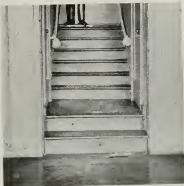
Fig. 2—The floor and stairs shown in Fig. 1 were found to have been gutted by these pests
