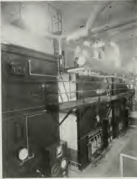
BOILER PLANT IN SUB BASEMENT TIMES BUILDING, LOS ANGELES
