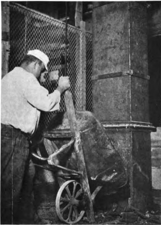
Workman dumping load of refuse down steel chute, the latter an innovation on building construction
