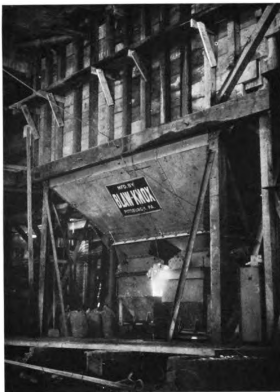
Concrete batcher in second basement. Materials were fed into it from bins in the first basement
