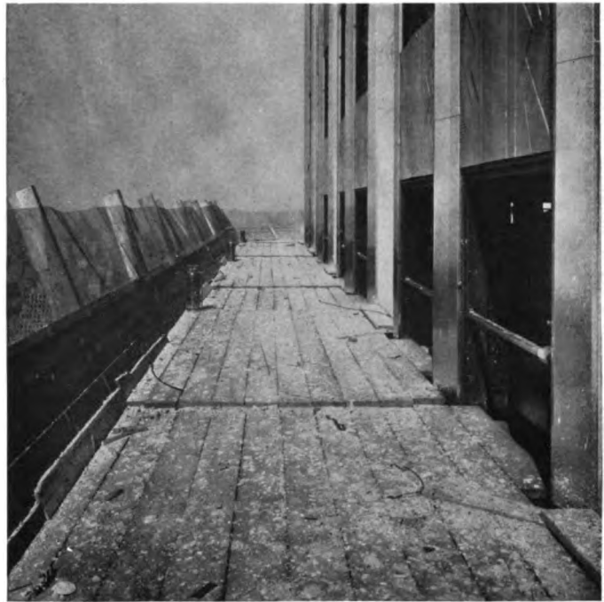
Section of catch-all. Note solid planking, the high guard of planks and wire, and fire extinguishers
