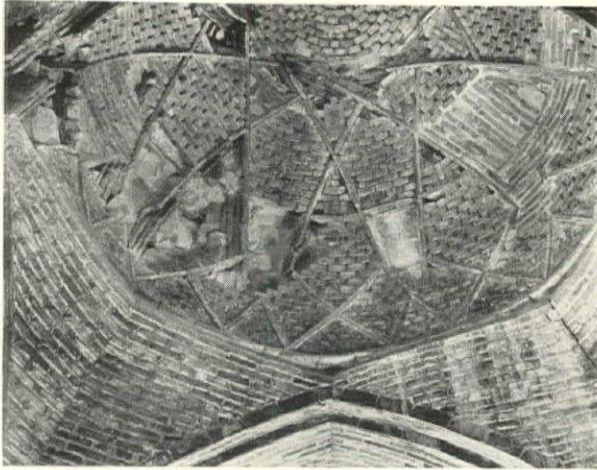
One of the more familiar type of honeycomb patterns found in the vaults of the Jami Mosque in Isfahan
