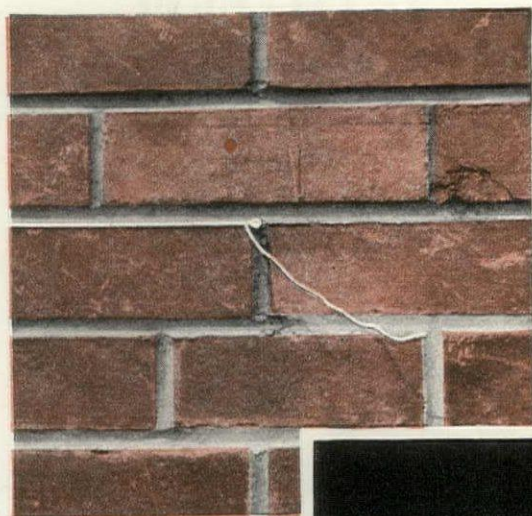
When a nail or line pin is used, the hole should be plugged with mortar as soon as the nail is removed.
