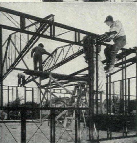
3 Roof trusses rise over wall structure. These two-section trusses are assembled during the erection procedure; truss is raised in place after sections are bolted together.
