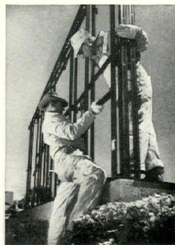
2 Wall section goes up on site. Wall section is welded at factory, arrives ready to be set in place. Wall structure is bolted to foundation.
