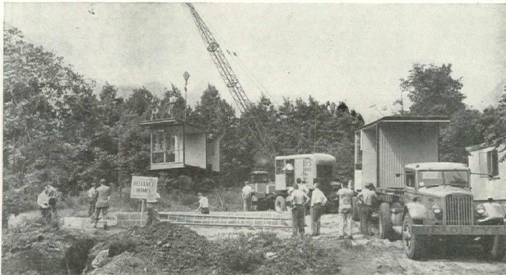
RELIANCE HOUSE arrives at site in seven completely factory-assembled units. Heating, plumbing and wiring are factory installed. House clips together in two hours. Floor and roof deck are light steel plates. Exterior walls are ribbed aluminum bonded to fiber board.
