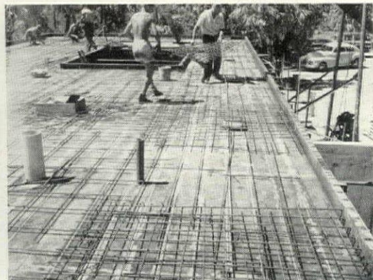
Reinforcing grids are put in place over welded assemblies atop column heads. The midspan rods are at same 1 in. level as plates of columns.
