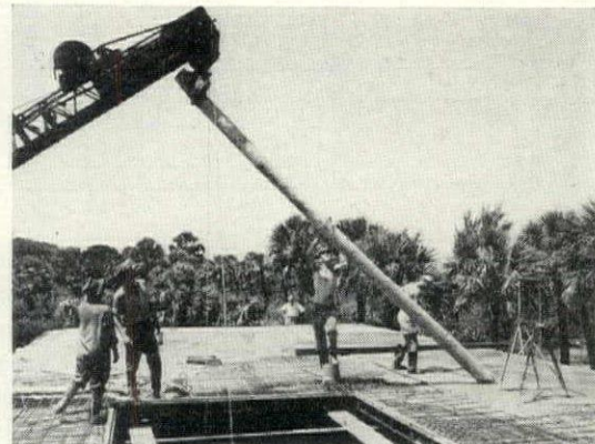
Pouring of roof slab is done with a specially designed, portable mixing and pouring rig which is built for great speed and ease in handling.
