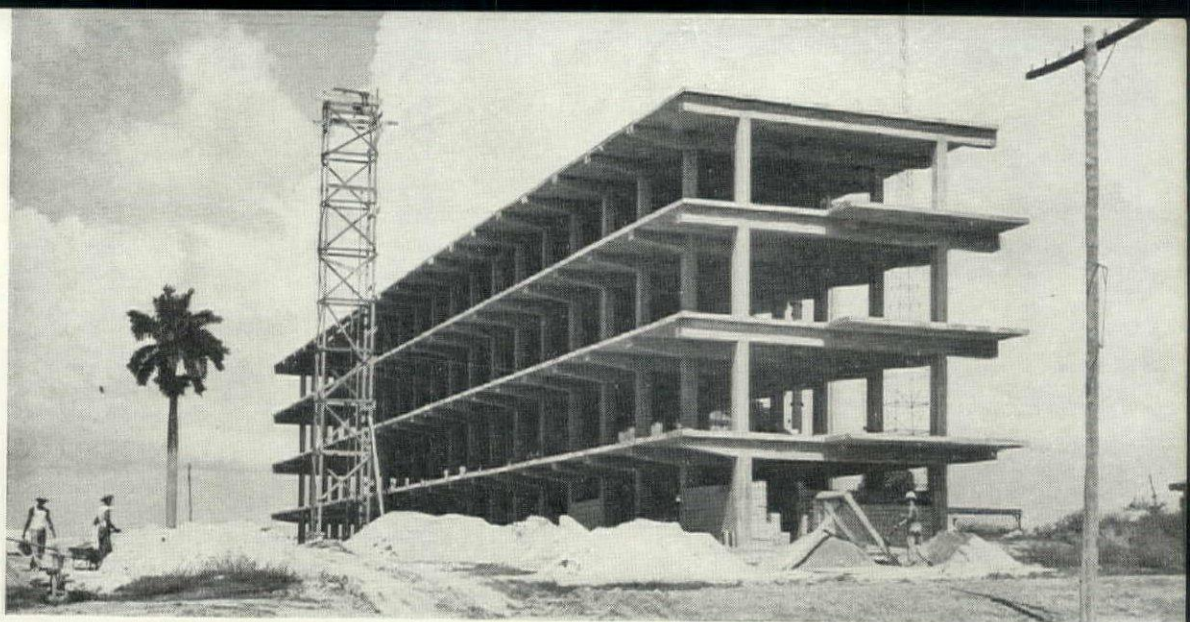
CUBA'S FIRST BIG HOUSING JOB is built in reinforced concrete, with concrete slab roof and marble flooring. Carpentry is Cuban hardwood. Kitchens are equipped for charcoal cooking.
