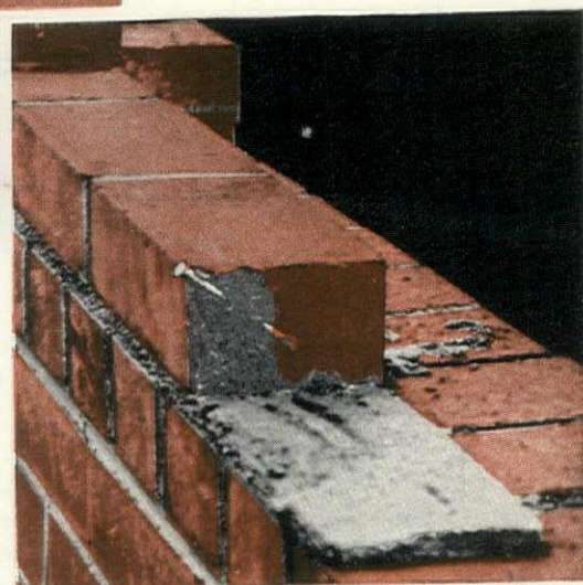
Water entering through the nail holes may travel through connecting voids and find an opening to the inside of the building.
