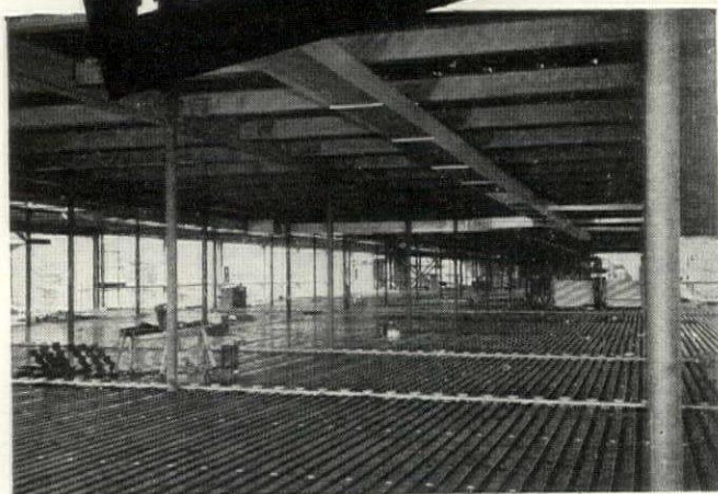
Q-Floor in place on first floor. Notice large number of cells—everyone available for wiring.
