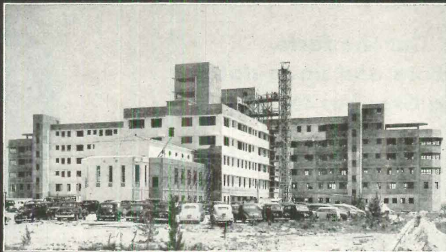
Mercy Hospital, Miami, Florida. Commencing of THOROSEAL applications. Architect—Steward and Skinner, Miami, Florida. Contractor—J. Y. Gooch Co., Miami, Florida. The finished THOROSEAL job is shown at the top of the page.
