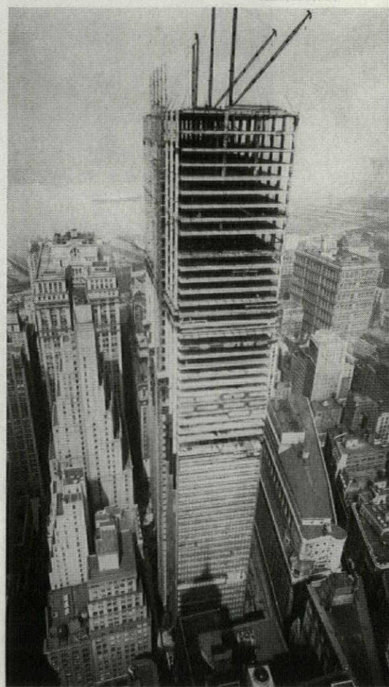
"TALLEST AND HEAVIEST" steel frame erected in the past quarter century was the boast made last month when the 60-story Chase Manhattan Bank Building in the heart of New York's financial district was topped out by Bethlehem Steel Co. ironworkers. The 53,000 tons of structurals for this 810 ft. tower are exceeded only by the 58,500 tons in Rockefeller Center's RCA Building and the 58,000 tons in the Empire State Building. The building's 40 main supporting columns each can carry loads up to 7,900 tons, or 50 per cent more than the Empire State's most massive columns. Architects: Skidmore, Owings & Merrill. Consulting structural engineer: Weiskopf & Pickworth.
