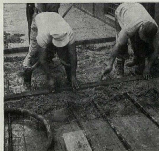
Illustration from booklet "Snow Melting and Ice Removal" shows steps in a sidewalk installation. For details on snow melting systems, write for this 32-page booklet.
