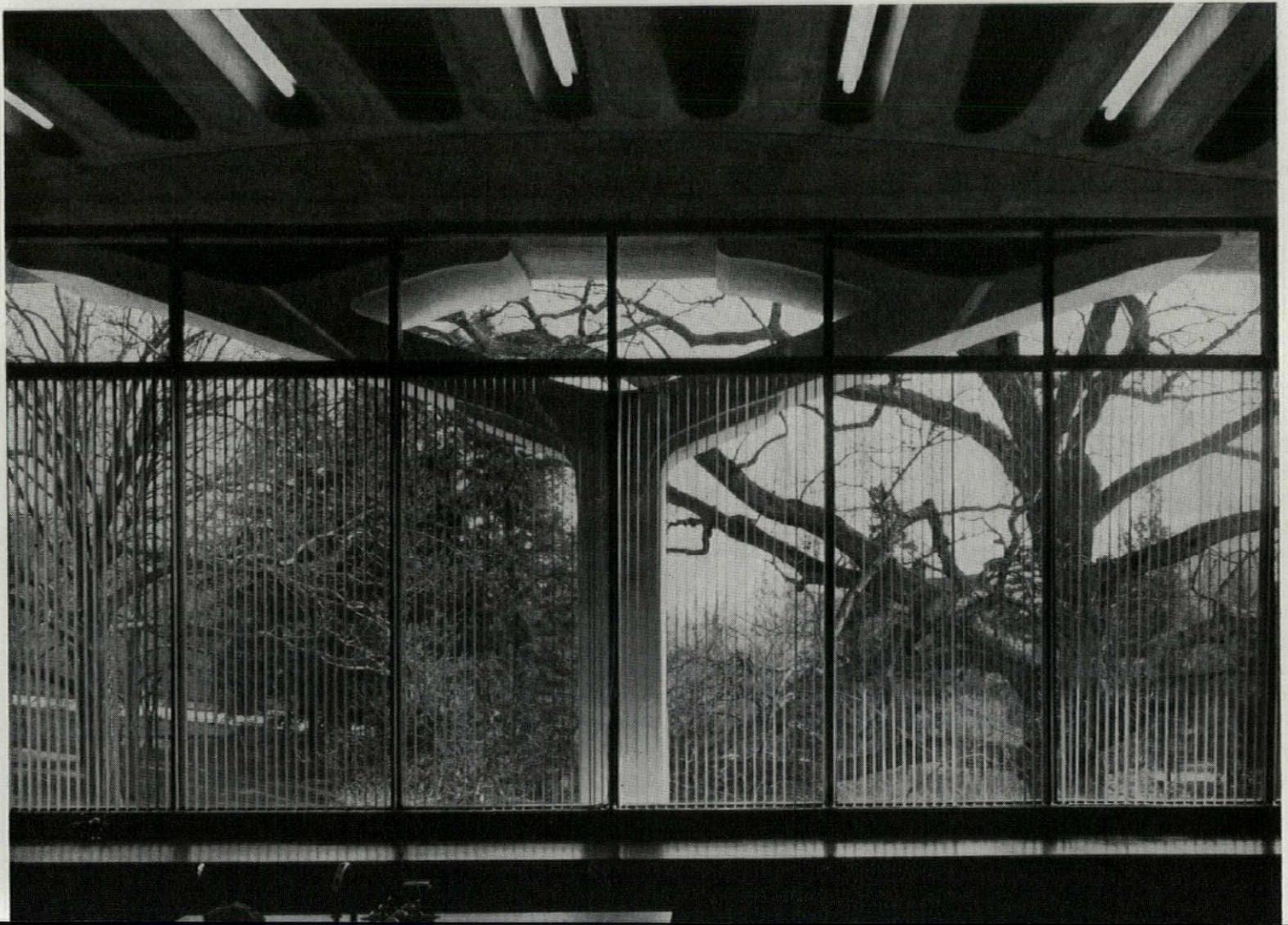
Curtain wall of precast concrete panels and steel-framed glass is set inside the column line.
