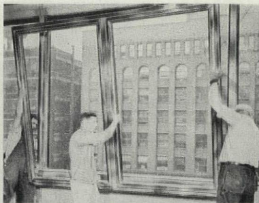
STAINLESS STEEL REVERSIBLE WINDOWS , here being installed at the Morton Salt Company Office Building, Chicago, Illinois, were fabricated by Republic's Truscon Division. Architects: Graham, Anderson, Probst & White, Inc. Contractor: Sherman Olson, Inc.
