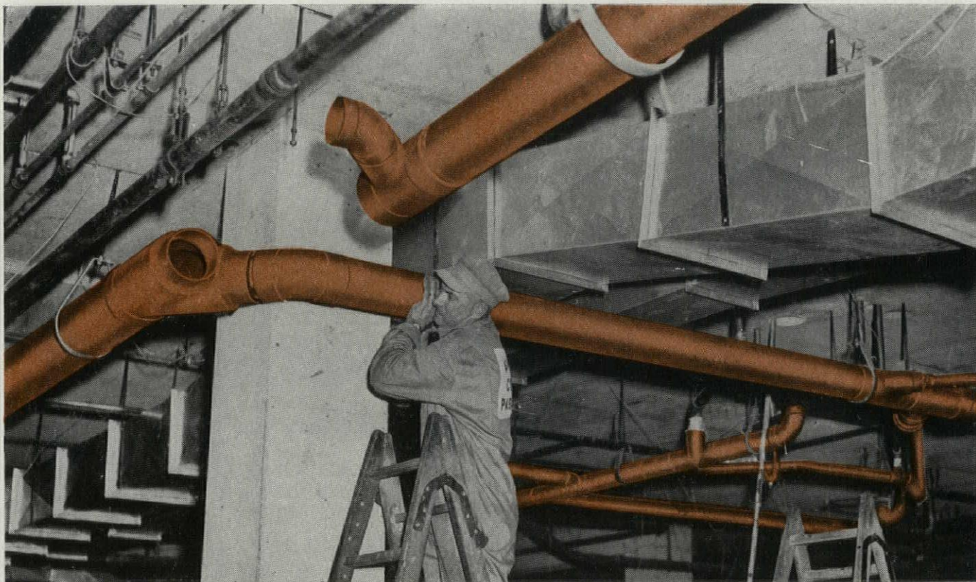
EASY TO HANDLE. Mechanic easily connects a length of 6-inch copper tube. More than 16,000 pounds of Anaconda Copper Tube, Type M, in sizes up to 8 inches, was used for the sanitary drainage systems. Architect and Engineer: California State Division of Architecture. Mechanical Engineer: Division of Architecture. General Contractor: Robert E. McKee, Inc., Los Angeles. Plumbing Contractor: E. O. Nay, Inc., Pasadena.
