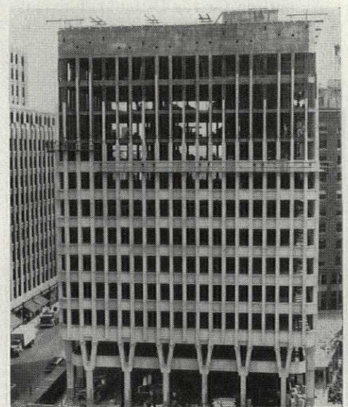
BOLD EXTERIOR COLUMNS of the Massachusetts Blue Cross-Blue Shield headquarters, nearing completion in Boston, serve a double purpose. They not only allow unobstructed interior space but also house the ducts for the high-velocity hot and cold air system. The Y columns at the base, and the building's chamfered corners are intended to emphasize the building's freestanding campanile character. Associated architects: Anderson, Beckwith & Haible and Paul Rudolph.
