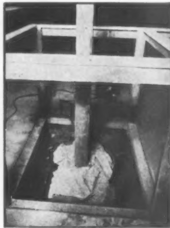
A thin wood column on loosely piled stones to support two floors and the roof; the poorest kind of construction
