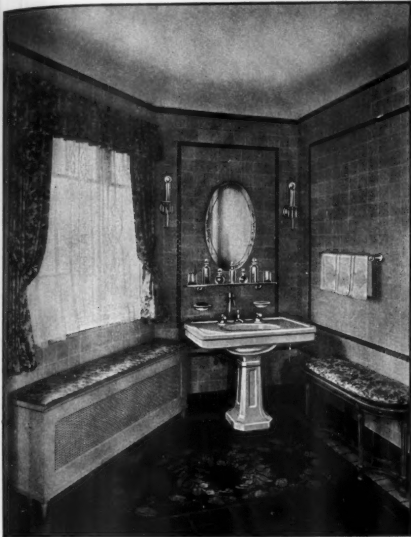
A corner of a small bath which may also be used as a dressing room, so attractively is it furnished and so carefully chosen is the plumbing
