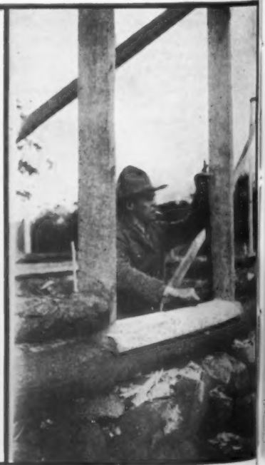
Leveling the door frames: one step that must be done with utmost care
