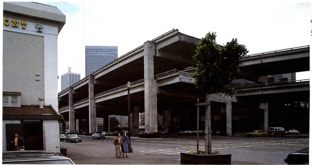
Section of the highway that would be demolished under the proposed scheme.
