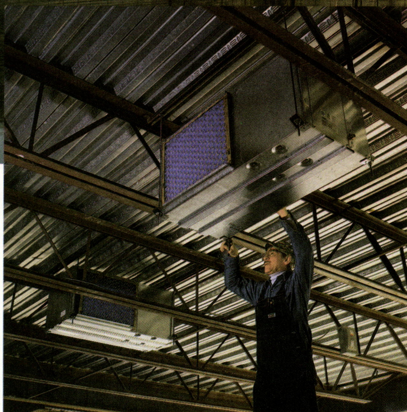
5-foot spacing between Vulcraft joists permits easy installation and maintenance of heat pump units.
