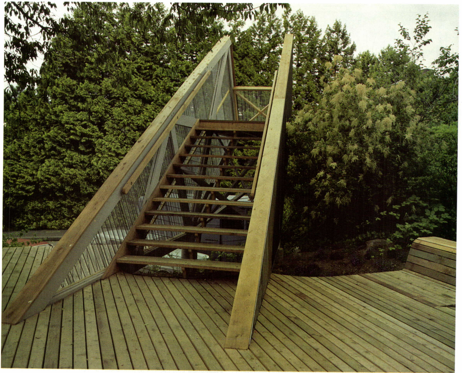
Facing page, top right, students building the 'Stairway to Nowhere' during a design-build studio taught by Steve Badenes of Jersey Devil. This page, the finished product.
