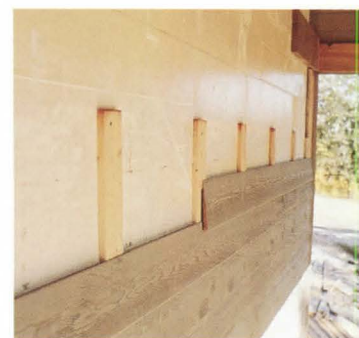
TOP: Openings in formwall are cut before concrete pour and are then framed to create doors and windows.
