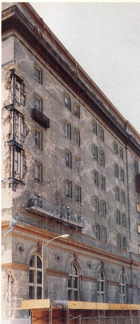
BEFORE: Hotel Oakland was damaged in 1989 quake.
