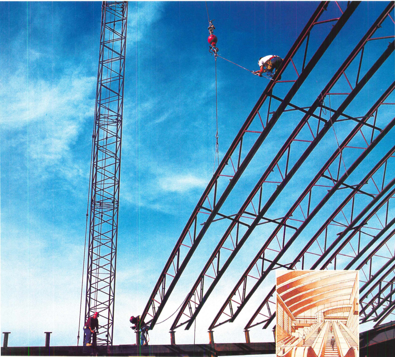
Arched chord joists top the Arrivals Hall, International Concourse, Hartsfield Atlanta International Airport
