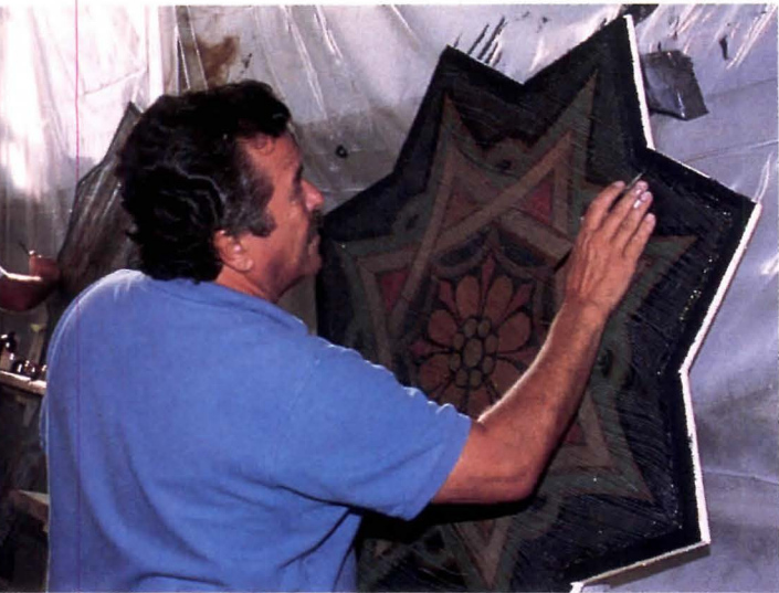
Craftsman (above) applies finish glaze to original star-shaped plaster ceiling panel. Mock-ups (below left) were created to test paints and glazes for reconstructed ceiling elements. Workers erected new steel-stud frame (below right) as substrate for restored ceiling panels.
