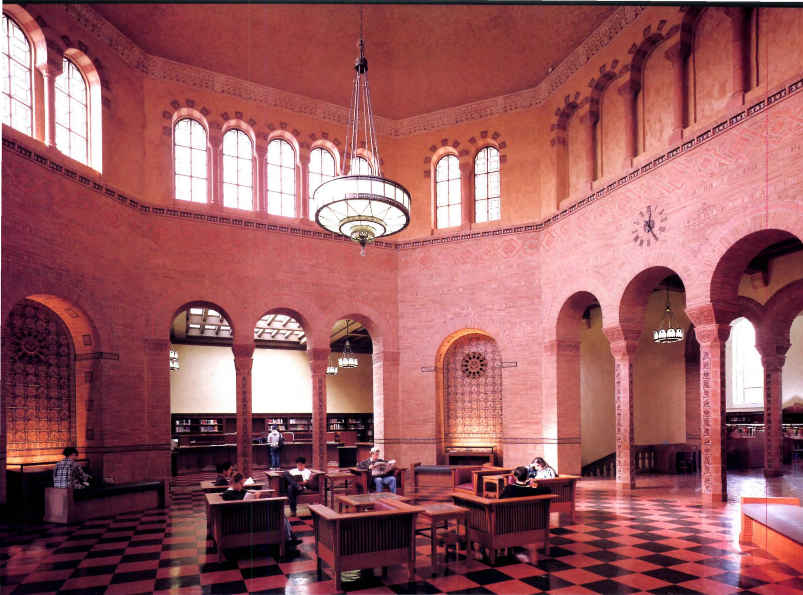
In rotunda, MRY reinstated brick, tile, and plaster wall finishes after adding shotcrete inside wall cavities.
