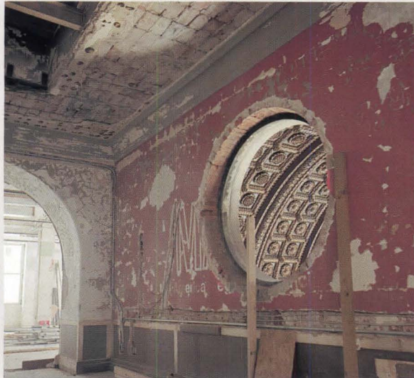
Photographs of second-floor lobby before (left) and after (right) show transformation of interiors. Plaster walls were patched and repainted.
