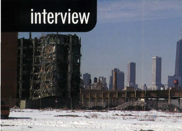
Chicago's Henry Horner Homes yield to the wrecking ball as part of HUD's HOPE VI program of public housing replacement.
