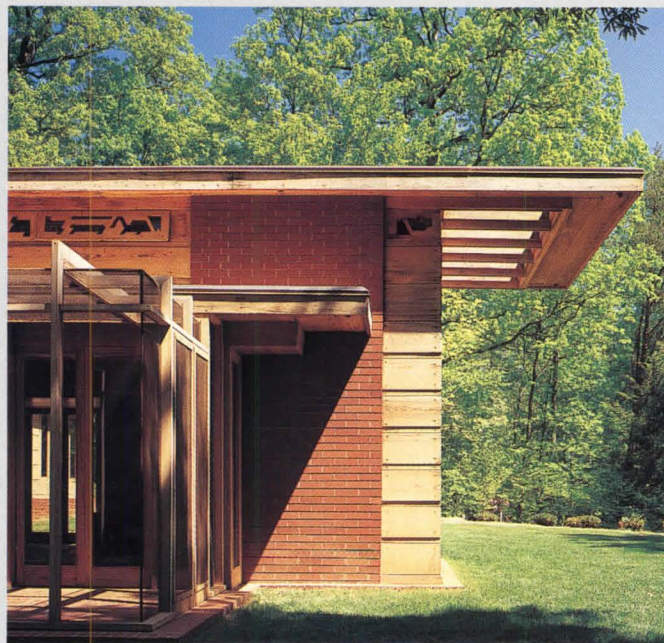
Quinn Evans reframed roof with laminated wood timbers, sanded and refinished original siding, and replaced all masonry. Weakened wooden roof supports between clerestory windows, which caused wall buckling, were replaced with steel rod-and-anchor configurations (drawing, far left), stretching from floor to roof.
