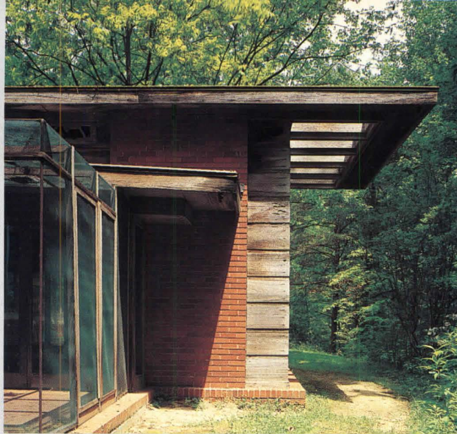
View of living room wing before reconstruction shows sagging cantilevers, sunken corners, and old cypress siding and masonry.
