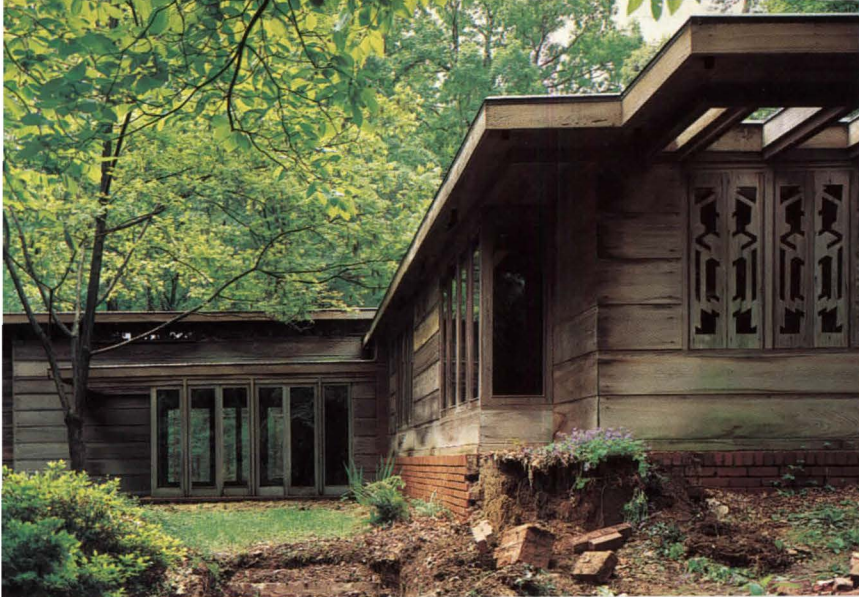
Badly damaged windows, planter, and cypress siding (left) were all restored (below).
