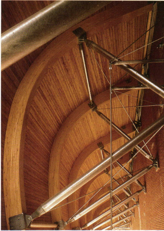
The coiving eaves of the middle hall's roof are held up with elegant V-shaped metal supports. The site plan (below) and sections and plans show the layout of the 1,200-seat theater (right top to bottom).
