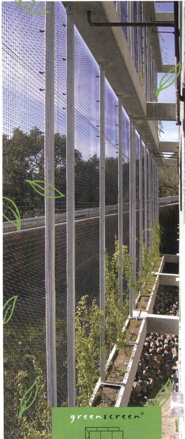
This 36,000 sq. ft. green screen facade on three five-level parking structures screens each south face, providing seasonal shade and important visual relief to this hillside site.
