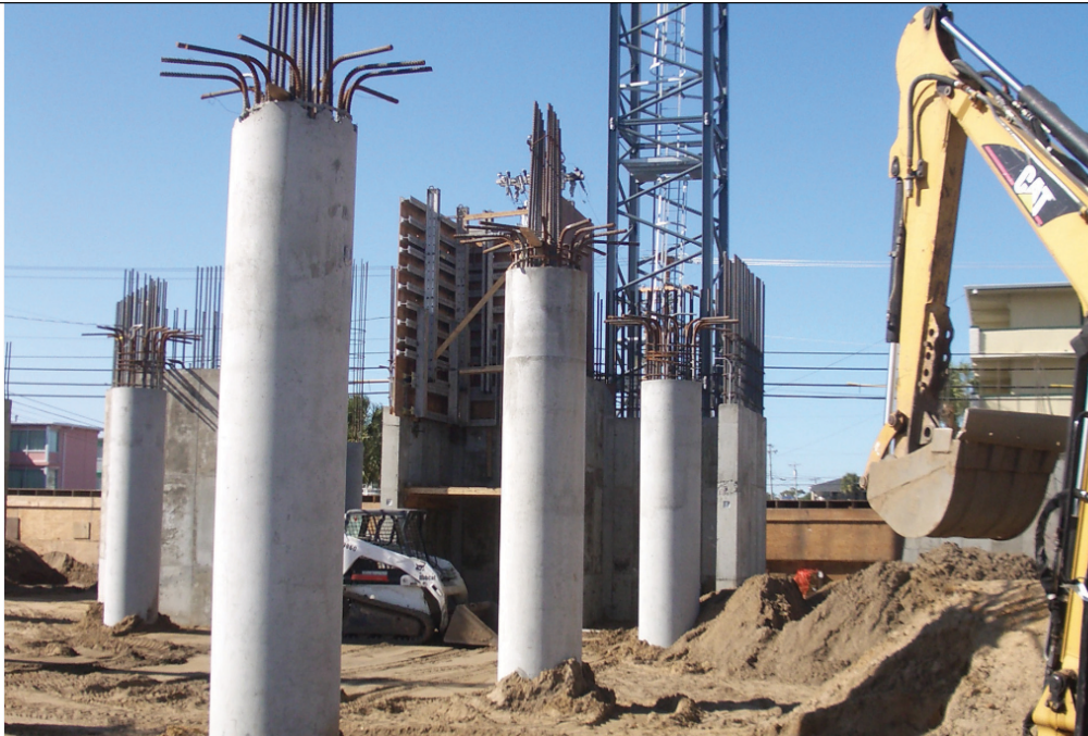
Column forms are often placed around reinforcing steel before concrete is pumped into the forms. After the concrete has set, the form is removed.
