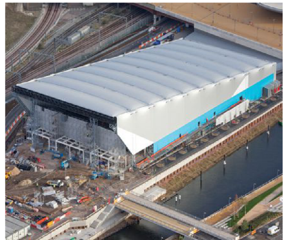
Water Polo Arena Wrapped in silver PVC and topped by an inflatable roof, the arena, designed by David Morley Architects, seats 5,000. The building will be deconstructed post-games; the seats and other components will be reused.
