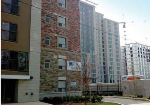
Finished and in-progress mid-rise multi-family buildings – all built with insulated concrete forms.
