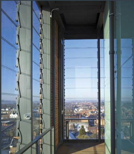
Louvered Facade Ventilators
