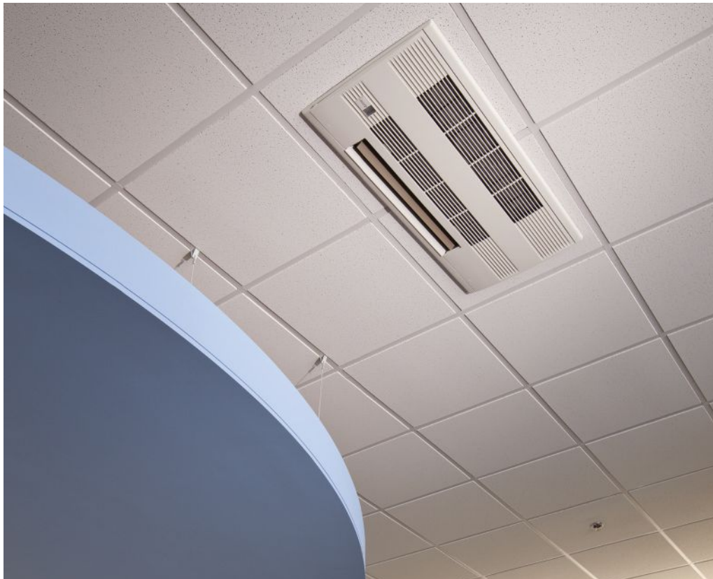
Ceiling-recessed indoor units offer a sleek method of air distribution in separate zones of a building's interior space.
