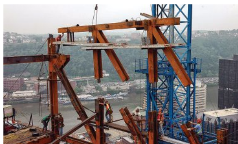
Shown during the erection of the structural steel frame, the new 33-story LEED Platinum Tower at PNC Plaza sits on a five-story podium and houses more than 800,000 sq. ft. of commercial office, auditorium, lobby, cafeteria, parking and amenity spaces. The superstructure is entirely steel-framed, using composite steel beams with a steel braced lateral system. In all, the project uses 8,000 tons of structural steel and 200,000 bolts. Photo courtesy: Sippel Steel Fab
