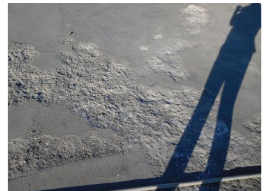
When exposed to elevated fire conditions, concrete is prone to spalling, as pictured here in this slab on deck. Photo courtesy of Wallace Engineering
