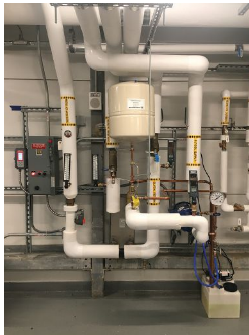
A snow and ice melt heat exchanger. Credit: Courtesy of Lily Helipads
