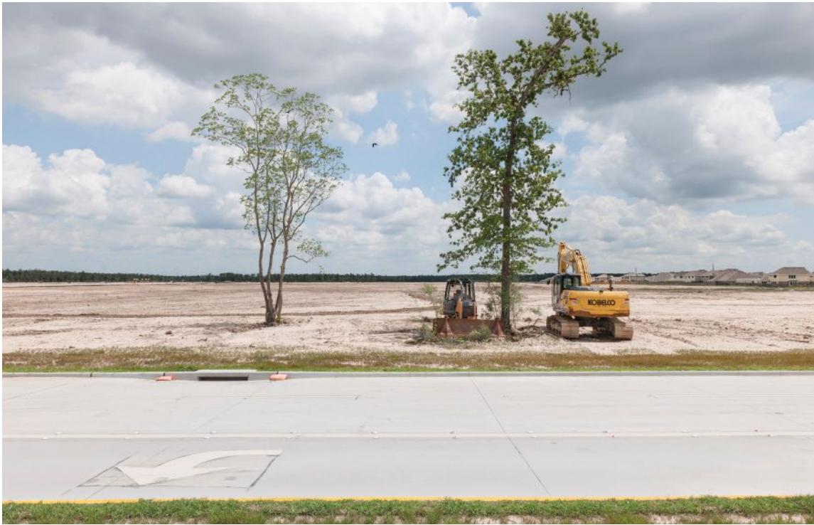
Construction recently started on a new development in Humble, part of Harris County
