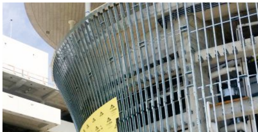
Steel Framing: Winning Project Phillip and Patricia Frost Museum of Science Aquarium Façade Miami Beach, Florida
