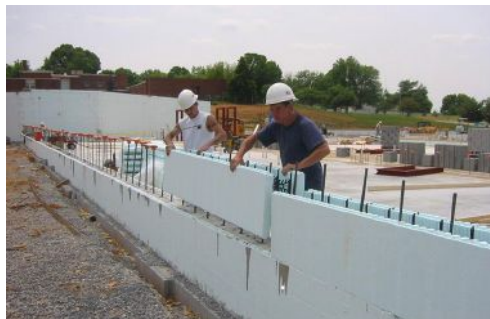
Richardsville Elementary School used the Nudura ICF system. Photo courtesy of Sherman Carter Barnhart.
