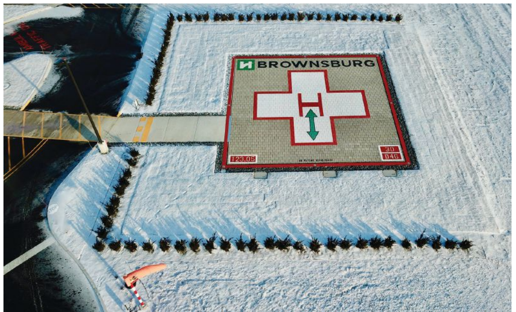
Automatic Snow-Ice Melt System at Hendricks County Regional Hospital, Brownsburg Indiana. Credit: Lily Helipads Stock
