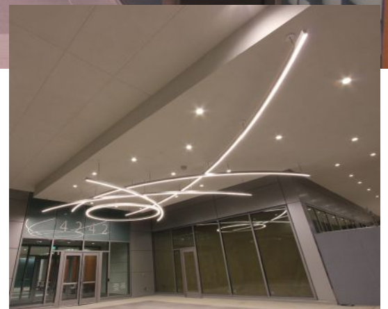
TANGENT Down™ • North Hills Tower II, Raleigh, NC Design: Cline Bettridge Bernstein & Duda Paine Architects
