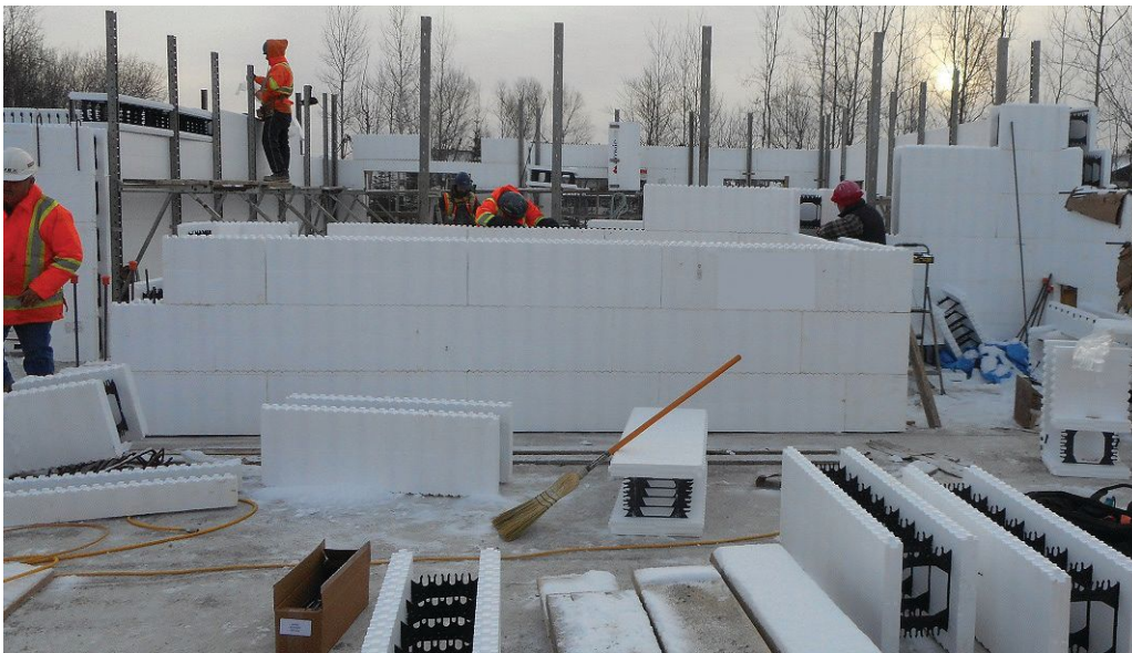
The starting of an ICF foundation wall. All the ICF forms and bracing are placed on the interior to allow for easy access and to expedite construction.
