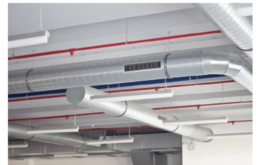
HVAC levels vary by zone and at certain times of day or year. Furthermore, this equipment does not generate a sound spectrum designed for speech privacy. CREDIT: © iStockphoto/Alexjay
