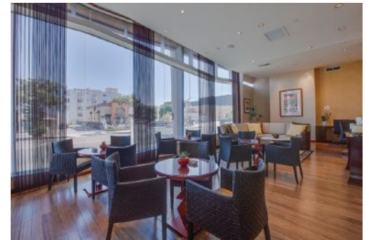
VRF in dining areas keeps both guests and staff comfortable, without interrupting the carefully-crafted ambiance.
