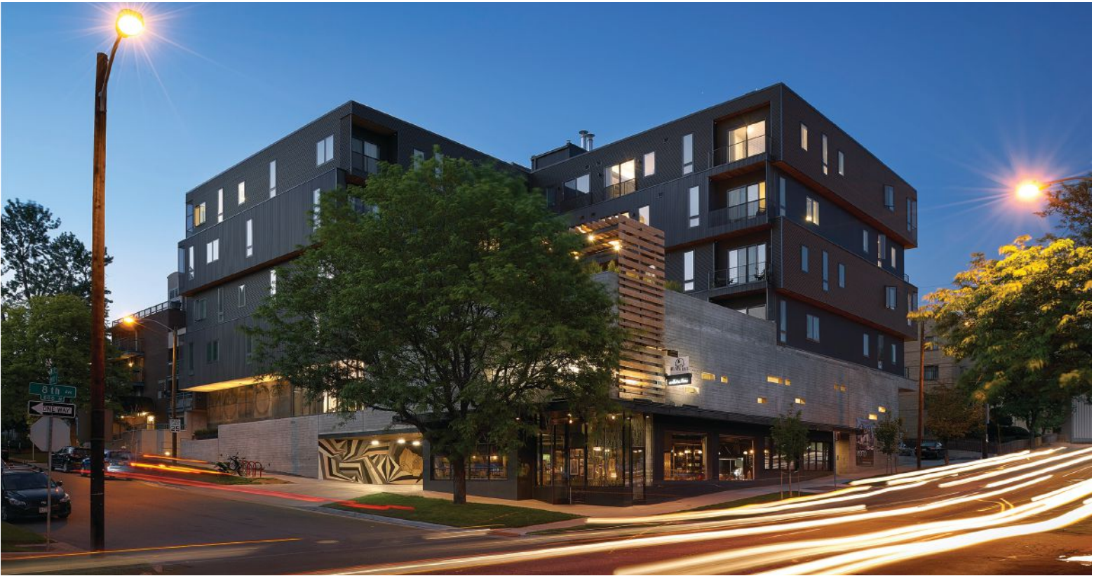
At MOTO, a panelized light frame wood wall system allowed each level to be framed in about a week and the entire project in less than a month. Photo: Ryan Gobuty
