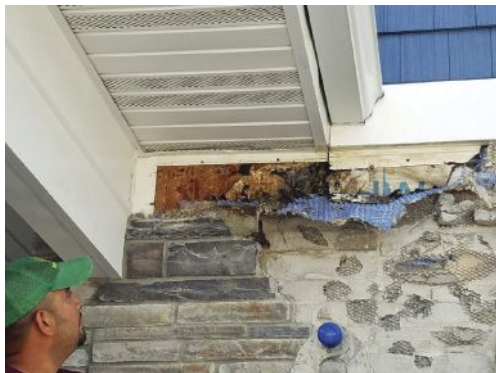
Figure 6. Example of a roof failure with no roof flashing... the rot underneath from improper horizontal transitions.
