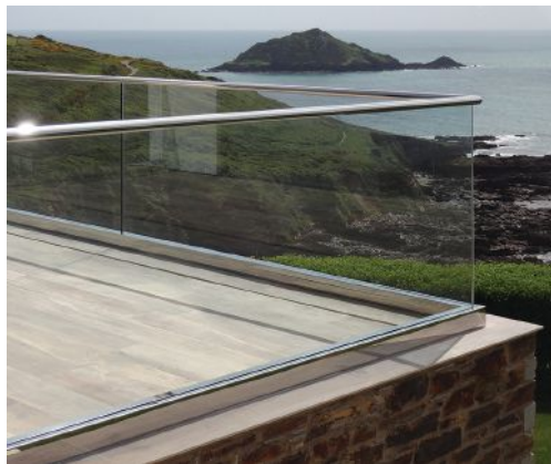
A glass railing system in a typical balcony application.
