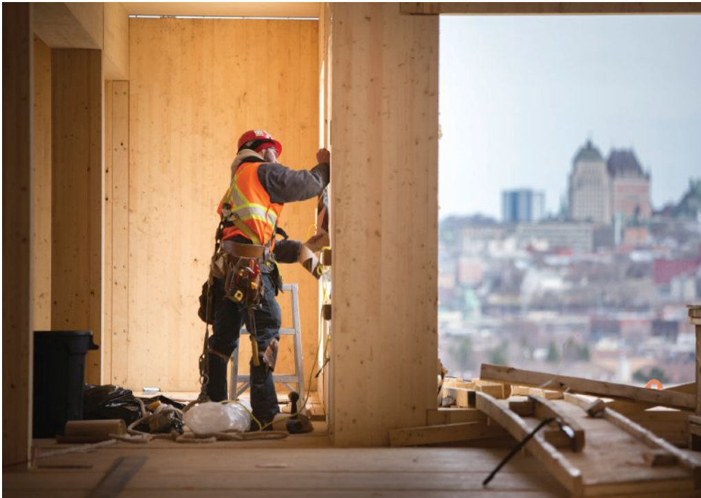
Mass timber's lighter weight boosted this Quebec-based multifamily project—dubbed Origine—by seven additional stories, giving it a total of thirteen. The same building in that location made from concrete would have maxed out at six stories high, given the low bearing capacity of the soil. PHOTO CREDIT: Stéphane Groleau ARCHITECT: Yvan Blouin Architect
