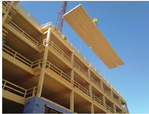
Mass timber products' light-weight advantage when compared to steel or concrete can often mean smaller foundations, helping to reduce a project's overall cost and seismic loads. T3 is 30% lighter than its equivalent in steel would have been, and 60% lighter than post-tensioned concrete according to engineer-led fabricator StructureCraft who supplied mass timber for the project | PHOTO CREDIT: Courtesy StructureCraft Builders DESIGN ARCHITECT: Michael Green Architecture (MGA) ARCHITECT OF RECORD: DLR Group
