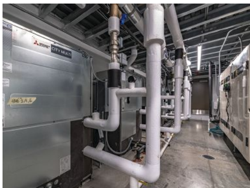
A geothermal water-source VRF system would save Fairway Independent Mortgage, headquartered in Madison, WI, $0.50–$0.75 per square foot in annual utility costs compared to a traditional hot water VAV rooftop system.
