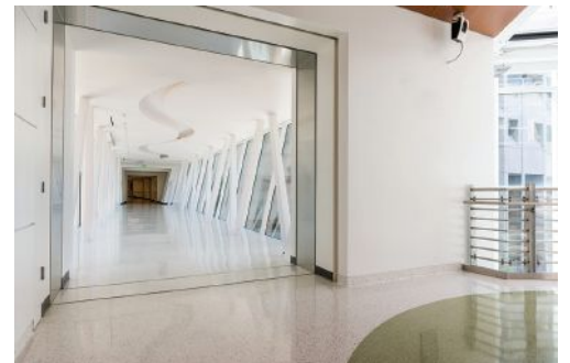
Zuckerburg San Francisco General Hospital, San Francisco, CA Caption: Zuckerburg San Francisco General Hospital must remain operational despite seismic events. Expansion joints allow the building to move 30-inches in every direction during an event.
