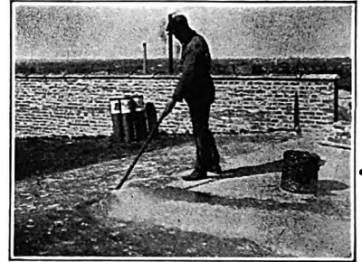
The concrete roof-deck is heavily mopped with a uniform coating of Barrett Specification Pitch.
