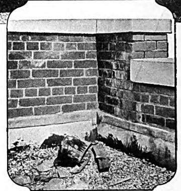
Close-up showing condition of metal flashings on St. Johnsbury Armory. No wonder the "roof" leaked!
