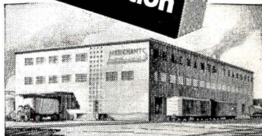
Top photo: View on 3rd floor showing 11'x17'-6" wall panel on platform ready for tilting. Above: Rendering of completed building. Brooks-Borg, architects; The Weitz Company, Inc., contractors.
