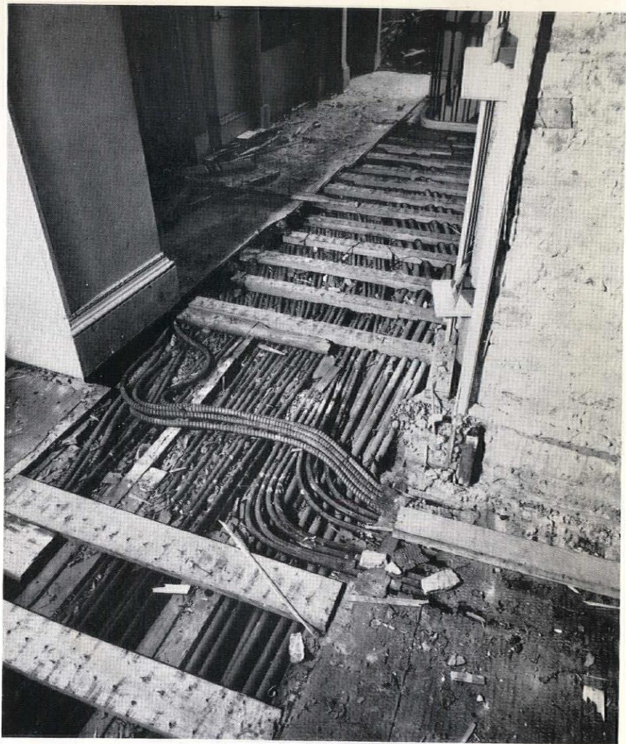
Conduits under the second floor of center hall. No wonder the floor squeaked.
