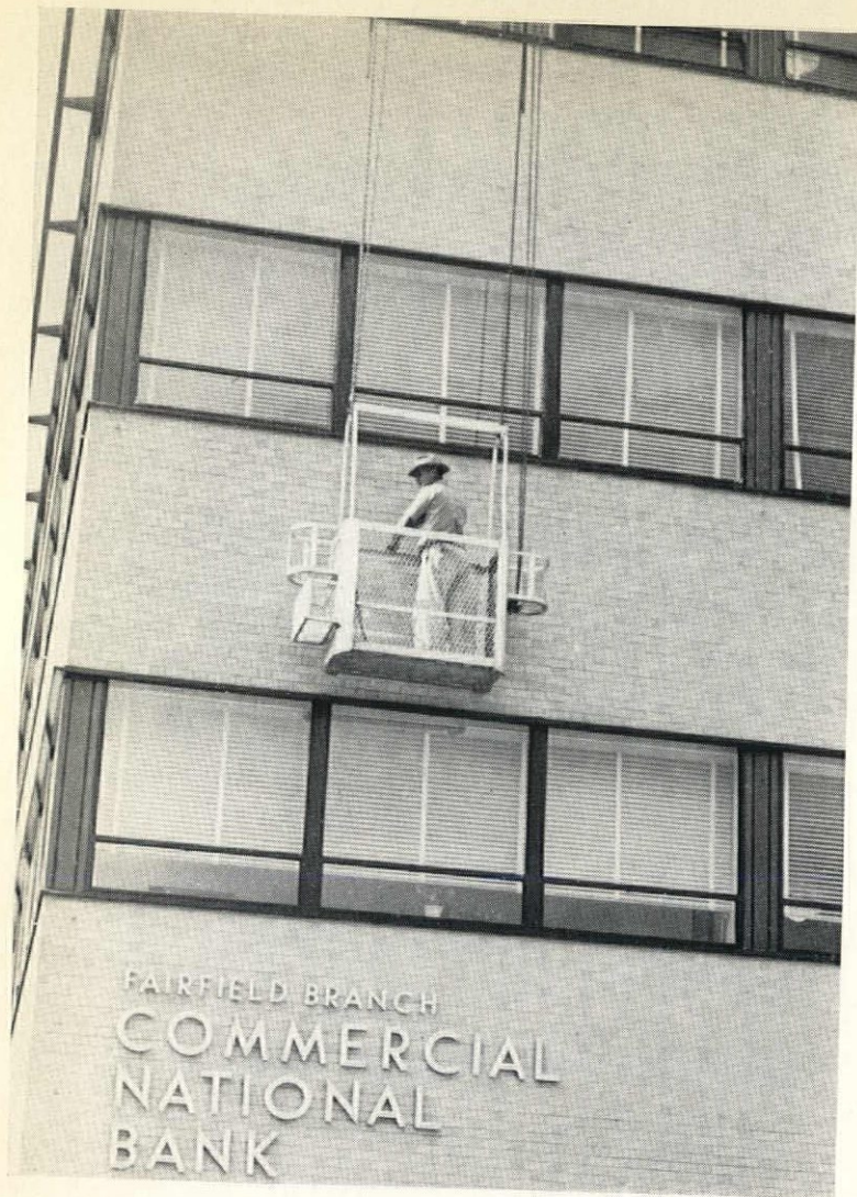
WINDOW-CLEANING DEVICE, FAIRFIELD BUILDING, SHREVEPORT, LA., SAMUEL G. WIENER, F.A.I.A., ARCHITECT
