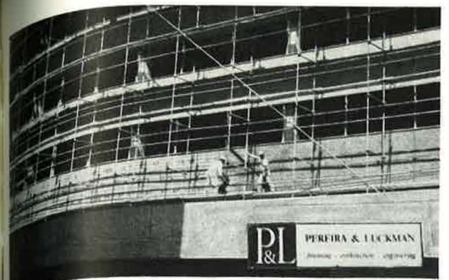
The 13-story Los Angeles IBM office building with K-LATH spandrel walls. Pereira & Luckman, architects.
