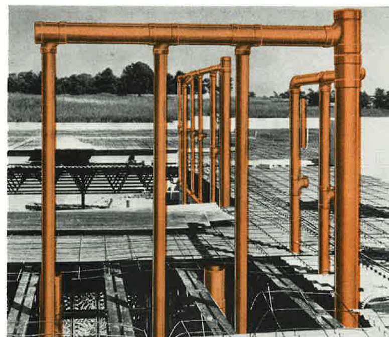
COPPER SANITARY DRAINAGE LINES for second floor lavatories at the Gower School. Light weight of copper tube and ease of making solder joints save many dollars on multiple installations like this. Compact assemblies eliminate wide plumbing walls, give greater usable floor area.
