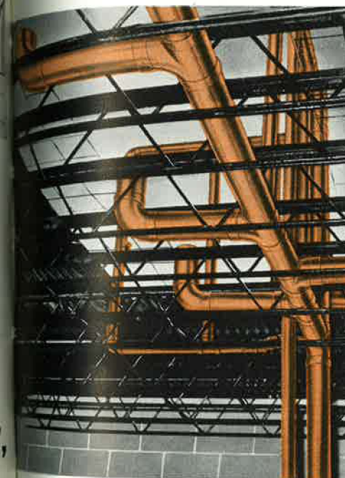
COPPER SANITARY DRAINAGE LINES roughed-in among structural members at Gower School. This space-saving installation would have been impracticable with heavy, threaded pipe requiring threaded or caulked joints.
