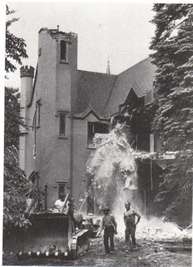
Despite efforts of preservationists, Bridgeport lost the mansion, a beloved local landmark, to the bulldozers
