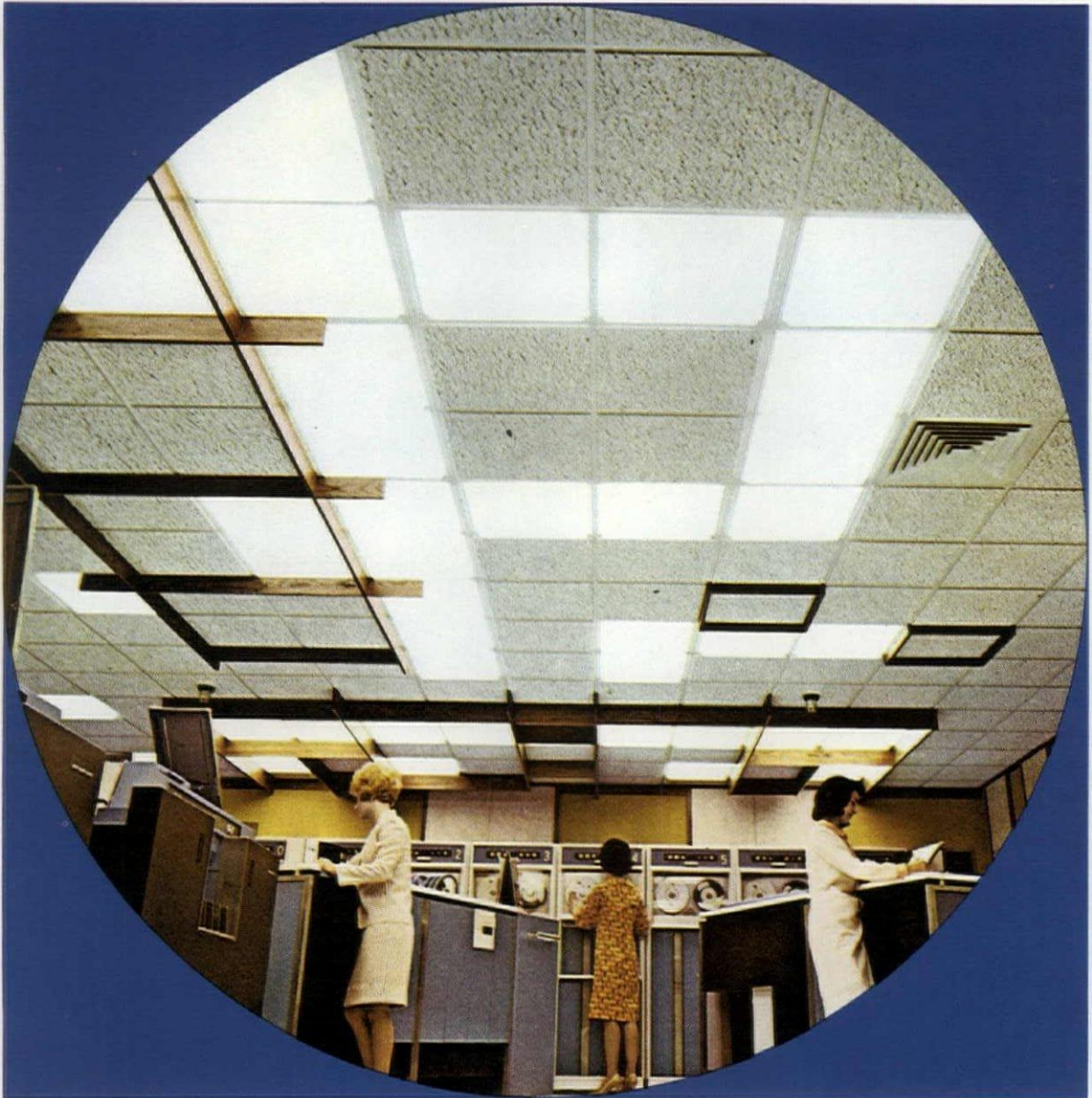
Data Processing Center, Continental Telephone Co., Wentzville, Mo./Architect: George Quick, St. Louis/Acoustical Contractor: Lindberg Acoustics, Inc., St. Louis.
