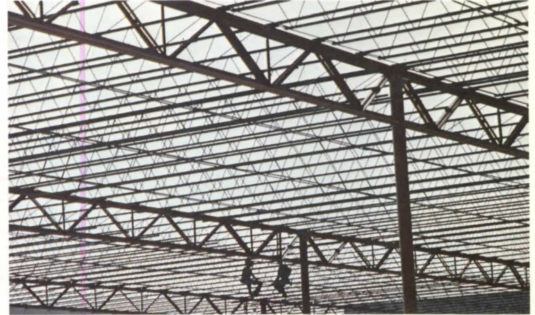
717 tons of joists and 433 tons of joist girders were used in this 746,852 square foot job.
