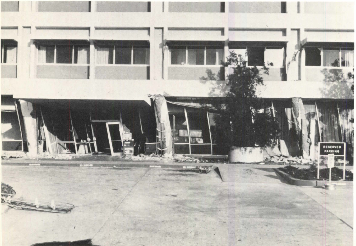
A rigid structure over an open first story offers this damage potential (hospital, San Fernando, Calif., 1971).
