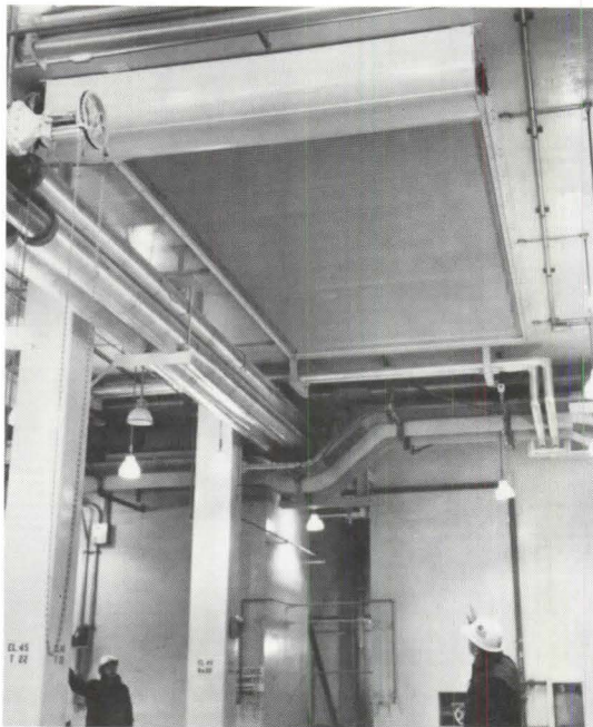
A J.G. Wilson A-9000 horizontal rolling door installation at Baltimore Gas and Electric Company, Calvert Cliffs, MD. The closure is motor operated, 12' wide x 24' long.
