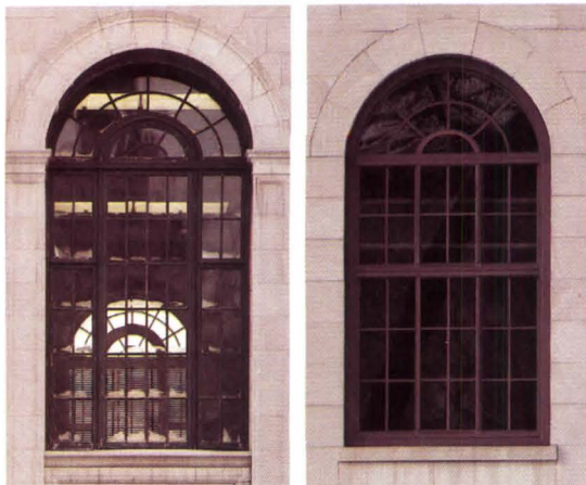
Required costly maintenance; old windows inefficient. Wide muntins cut visibility.
