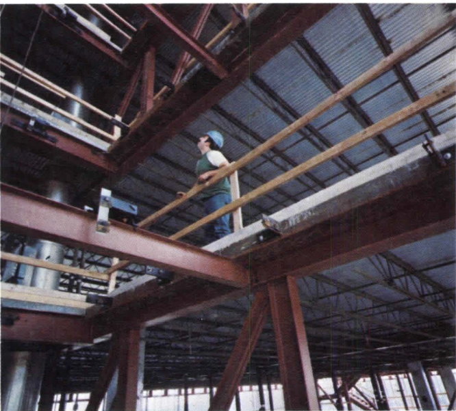
Interior view during construction shows large, column-free spaces. Typical bays measure 53 ft 6 in. by 22 ft. Bethlehem supplied 700 tons of structural steel for the project.
