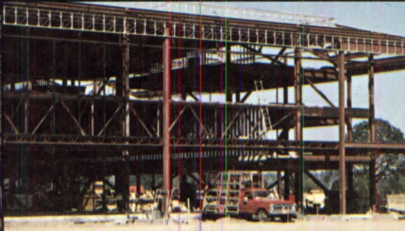
The versatility of designing with Vulcraft steel joists and joist girders helps meet complex design requirements like this unusual eight foot interstitial floor space.
