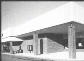
Giant Foods Shopping Center, Baltimore, Maryland. Architect: Coupard & Associates. Manufacturer: Cem-Fil Corporation, Nashville, Tennessee.
