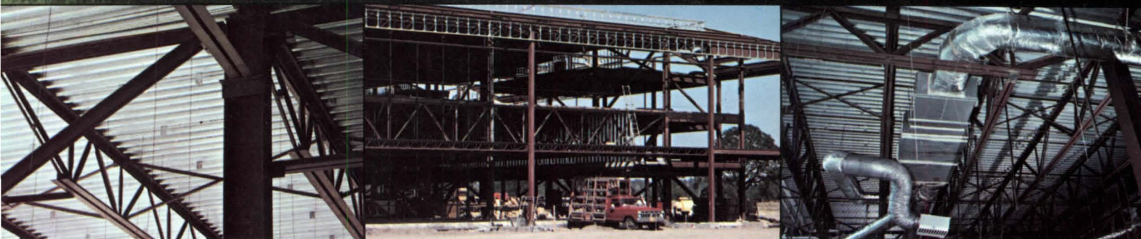
The Hewlett-Packard facility in Cupertino, California, the first of six to use the Vulcraft system.
