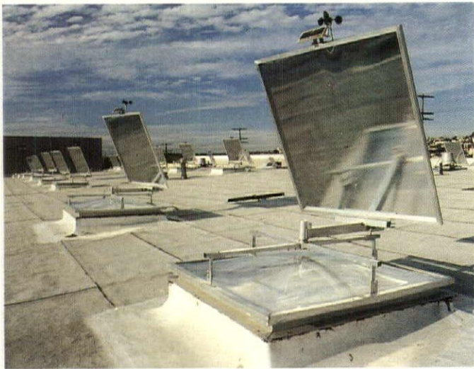
A mirror mounted on a heliostat projects a fairly constant beam down into a skylight.
