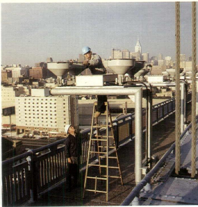
Workers for W.V. Pangborne Company, the contractor that installed the bridge lighting system, check a luminaire.
