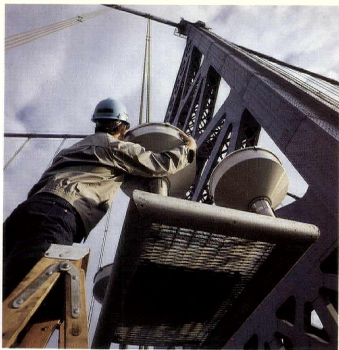
The luminaires' target is the catenary cable that supports these 200-foot-long suspender cables.
